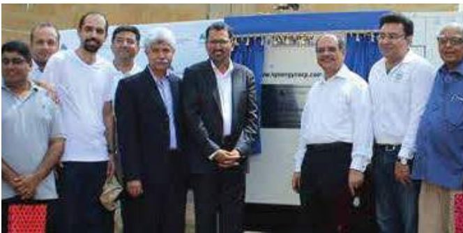
Mr. Ali Sultan, Group Head, Treasury & FI, Bank Alfalah Limited, inaugurated the 60 kv Generator donated by Bank Alfalah to CDSS. On this occasion Bank Alfalah staff and CDSS management were also present.
